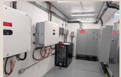
Battery storage room (exterior and interior)
